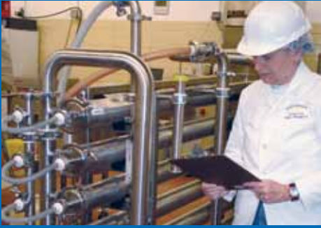
Membrane filtration equipment at the WCDR.
